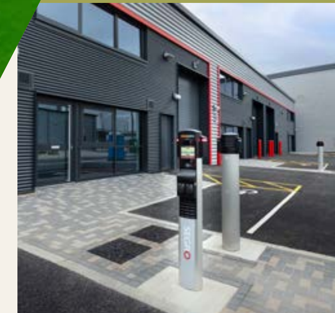
EV charging points
