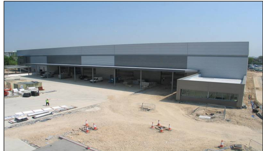
DB Schenker at the Portal Site, Heathrow Due to be completed August 2012
